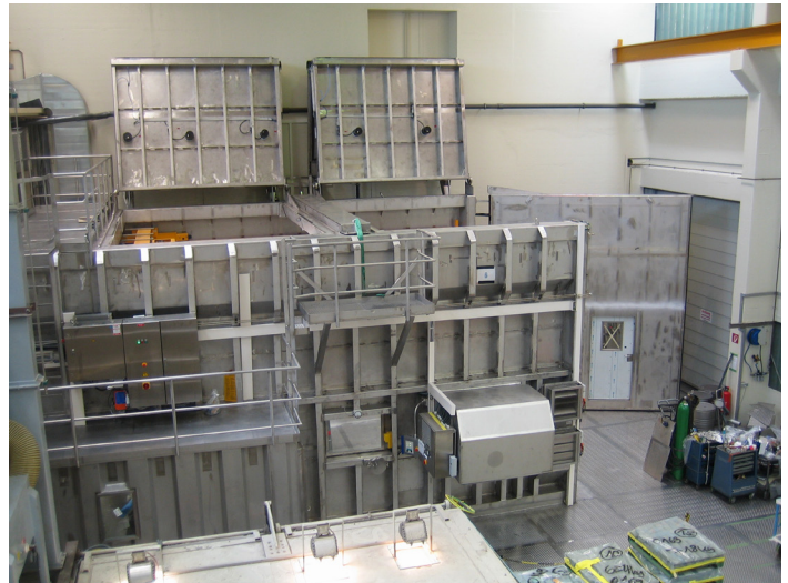
Example of a multi-function box (e.g., segmentation, workshop, decontamination) with foldable roof opening
