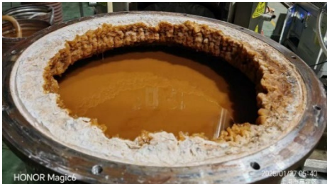
Salt crystallization at drum inner walls, bottom and liquid surface.
